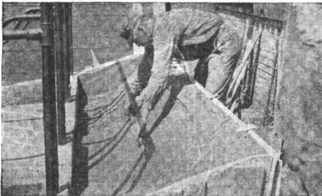
7. Manger templates are strips of iron about 1/2 in. x 2 in. bent by any blacksmith to hang from top of curb to top of manger form. A light strike board is then dragged from the curb to the top of manger form, riding on the templates which are then removed before the concrete hardens. The Manger should be finished with a metal trowel.
